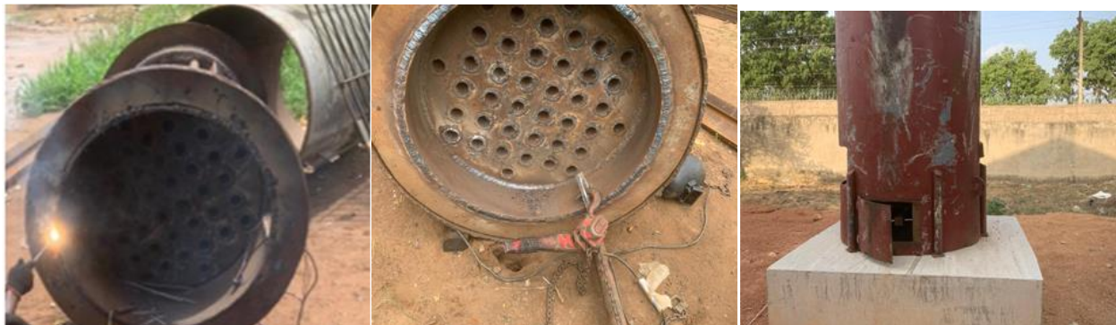
Figure 2: (a) Welding of the combustion chamber to the inner shell. (b) The welded assembly part is ready to be lifted. (c) The steam boiler on fabrication
